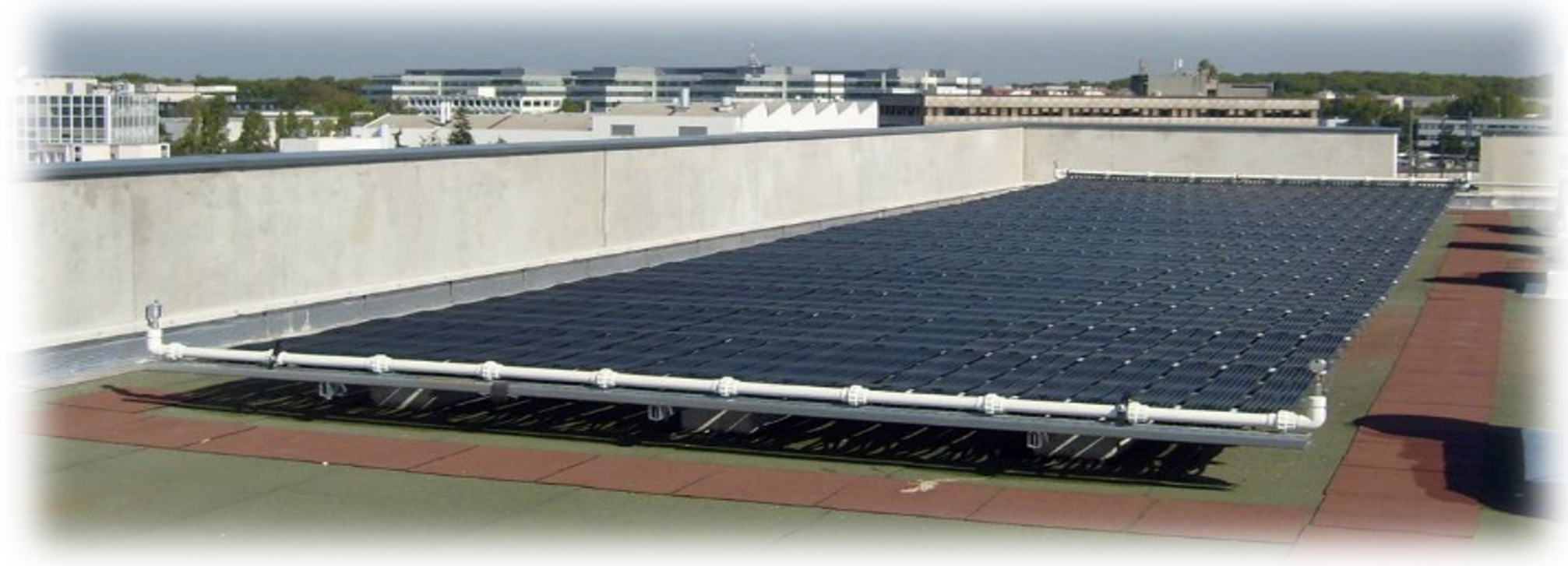
Flexible collectors on a roof
