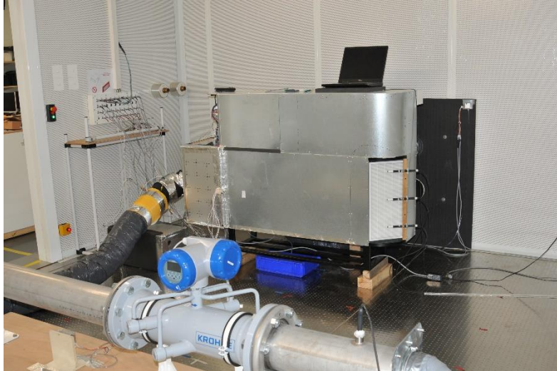
The AHPP has been installed inside the Internal Climate test room which simulates the ambient conditions of a room in a building
