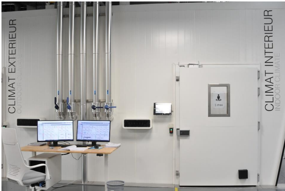
France Energie laboratory with 2 test rooms.
