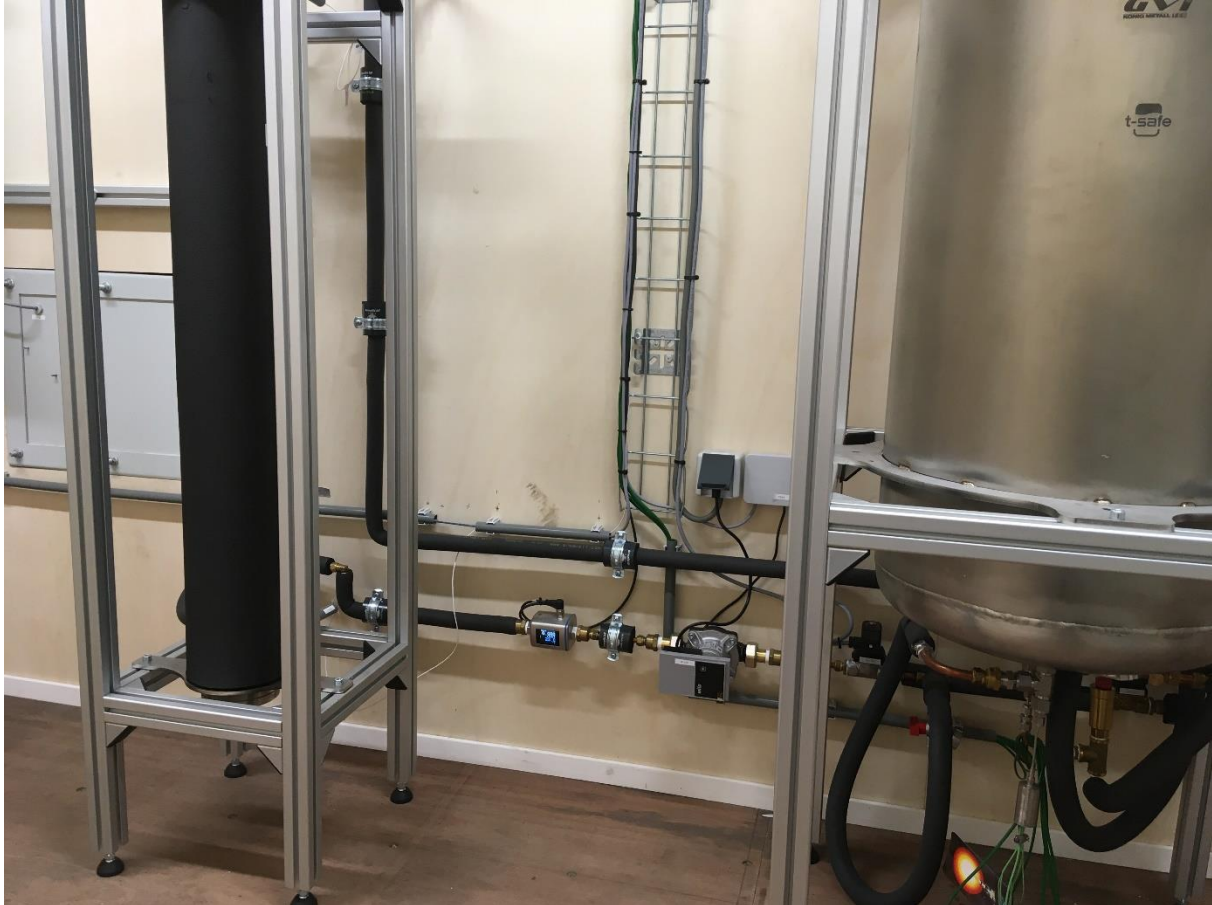
Figure 8: Flow meters and pumps between the CLC Emulator Demo Reactor and the MRSU.
