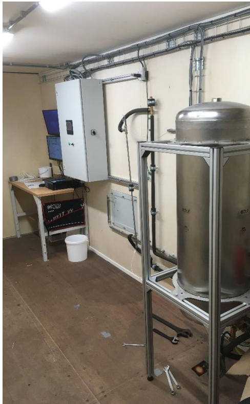
Figure 5: Day 9 of construction. Note: CLC Emulator Demo Reactor was not yet received so the system was tested using a bypass instead.
