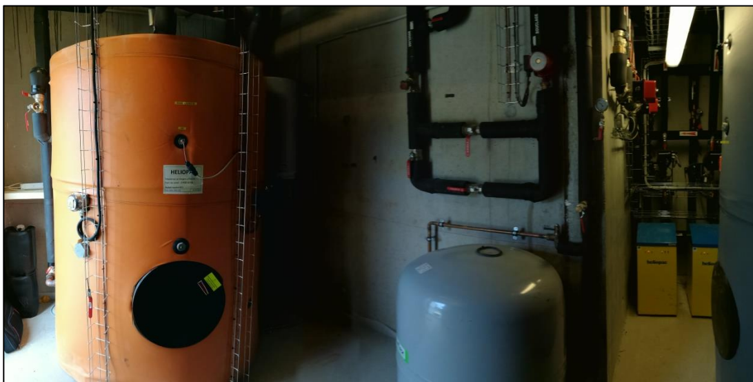
The third buffer in orange and the expansion vessel in grey.
