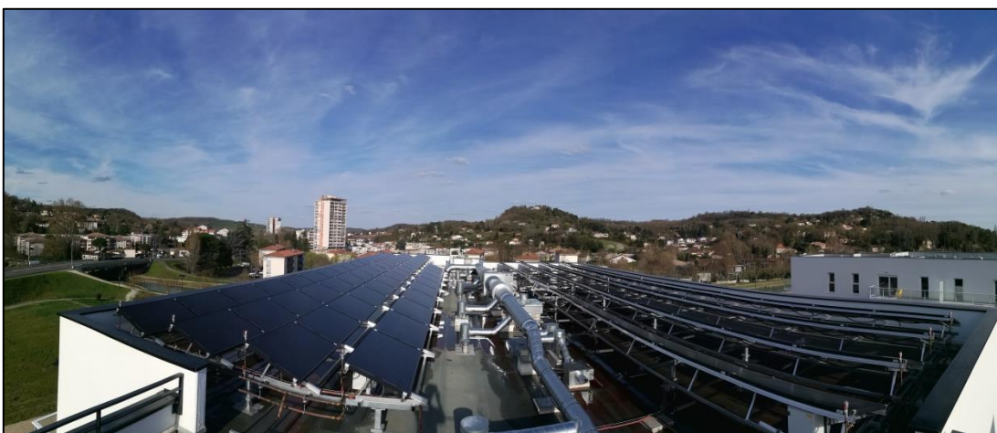
PVT solar panels
