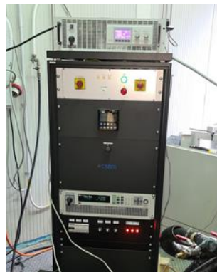
DC bus generator
