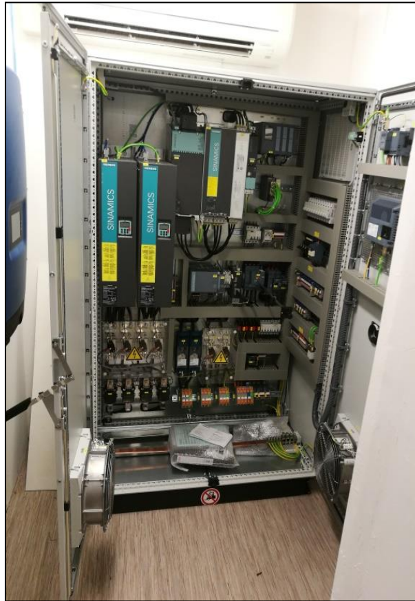
Figure 13 : Photo of the Electricity converter system (ECS)
