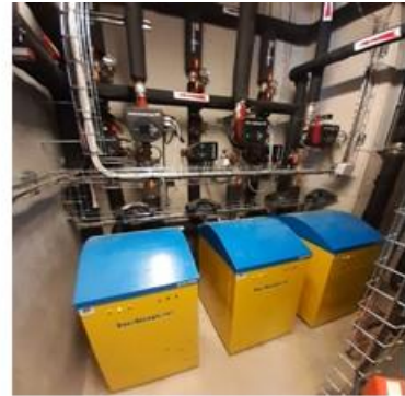
W/W Heat Pumps (3*12 kWth)
